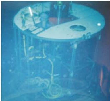
Figure 1. (above) Photograph of sub-sea station offshore Japan taken from Dolphin 3K (remotely operated underwater vehicle, "ROV"). The cylindrical superstructure sits on top of the re-entry cone and houses the power supply, recorder unit and controller unit for the borehole sensor package embedded 110 m below. ROVs periodically make electrical connections to communicate with the station, exchange the data recorder, and update the system.
